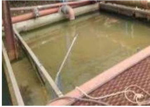
Gambar 3. 18 Sludge Tank PT Z
